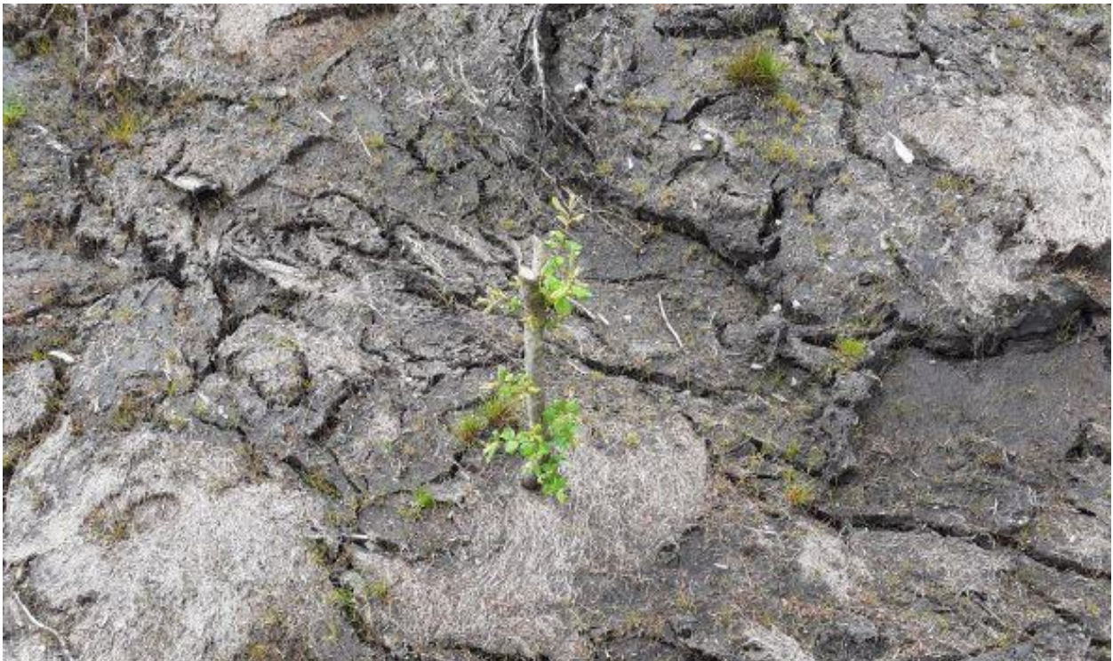
Photo 3 – sapling growing in area where wall 2 was located, 8/7/22
