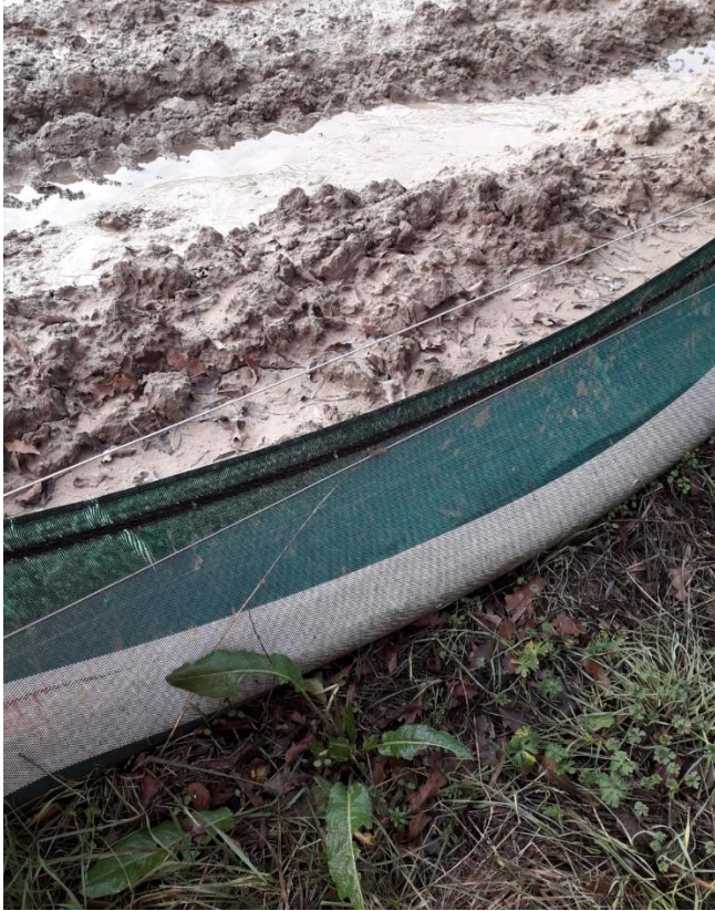
Figure 5.7 Terrastop silt fence properly buried into ground surface acting as effective silt barrier
