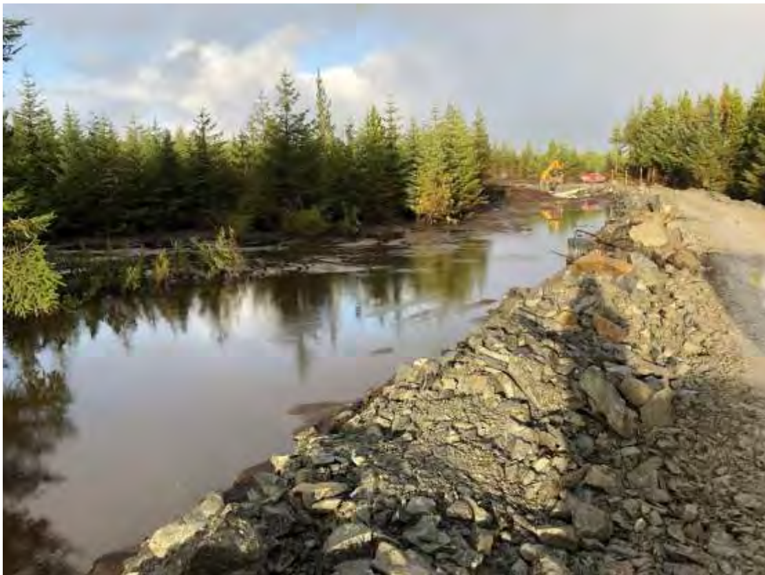
Figure 2.2 Water and sediment impoundment area upstream of Wall 1 showing stabilised situation and deposits of peat up to surface of water
