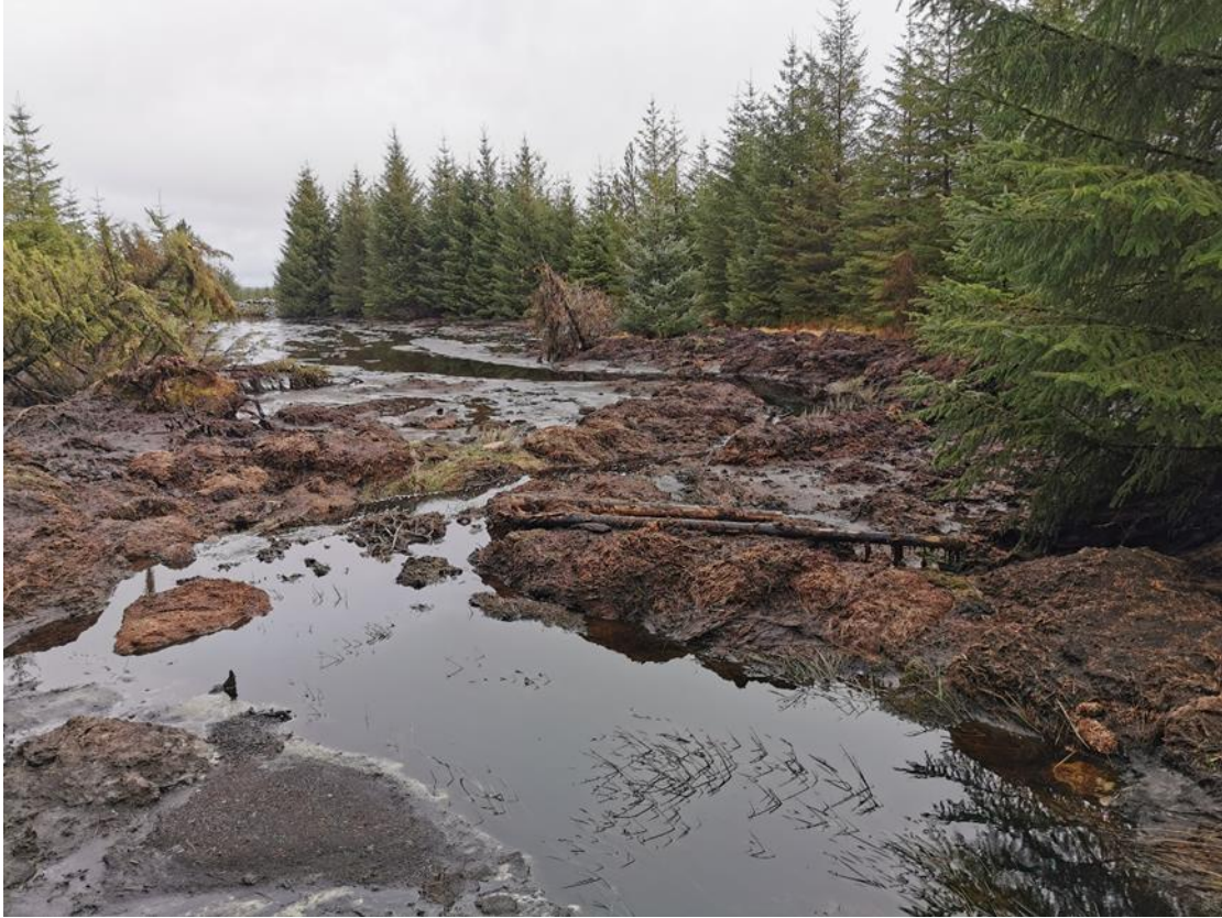
Plate 2.3 View of impounded area prior to commencement of sediment removal works, facing downstream
