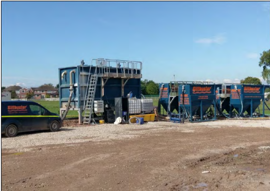
Figure 5.12: MT30 Chemical Pre-Treatment system with 4 No Lamella clarifiers
